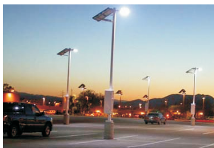
LED Bulbs Used as Streetlights
